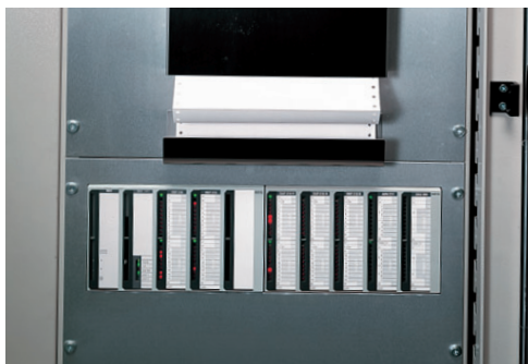
PLC BRANDS: SIEMENS, ALLEN-BRADLEY, MODICON, MITSUBISHI
