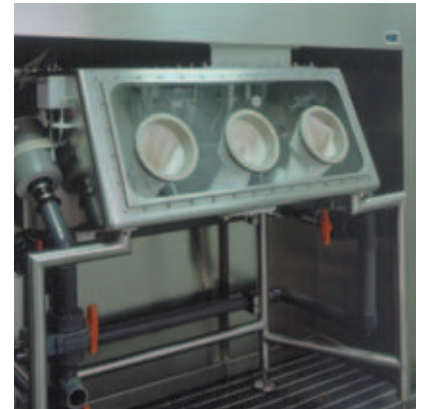
UNLOADING SIDE WITH ISOLATOR
